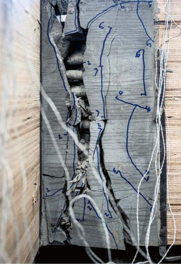
One of the cracks induced by extreme loads is several centimetres wide.
