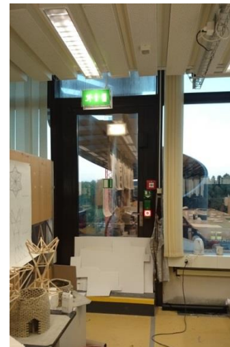
Blocked escape door
