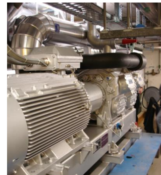
Heat pump for the use of waste heat
