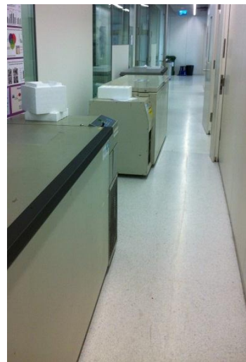
Obstructed escape corridor
