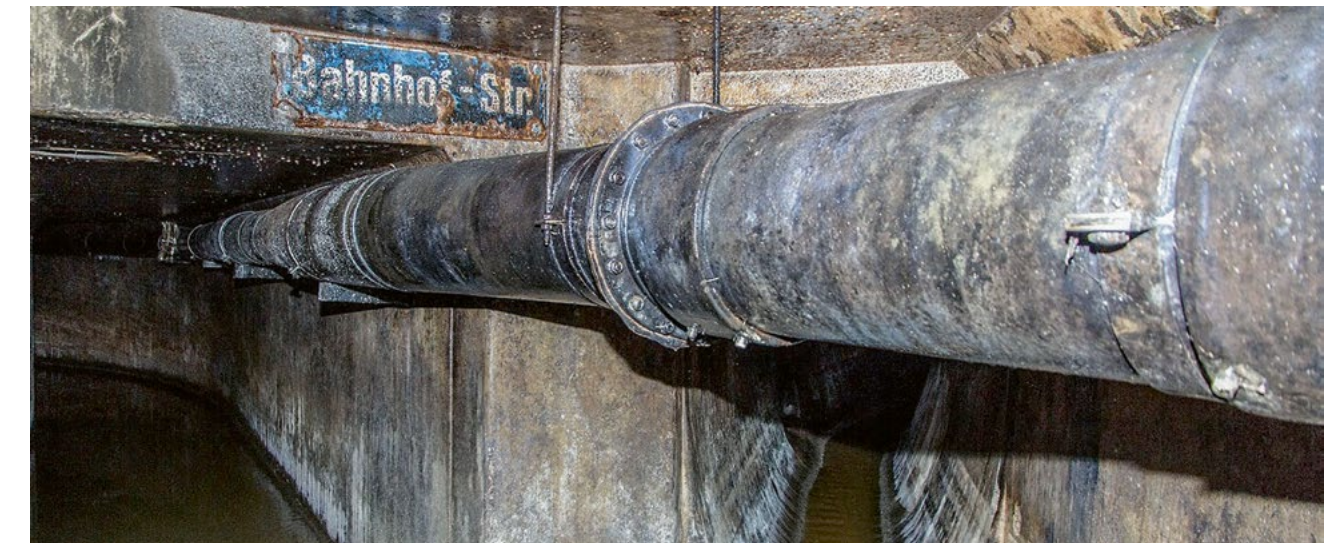
↑ Beneath the Bahnhofstrasse in Zurich, a sewer conveys wastewater to the treatment plant. Rainwater is channelled through a separate pipe.
