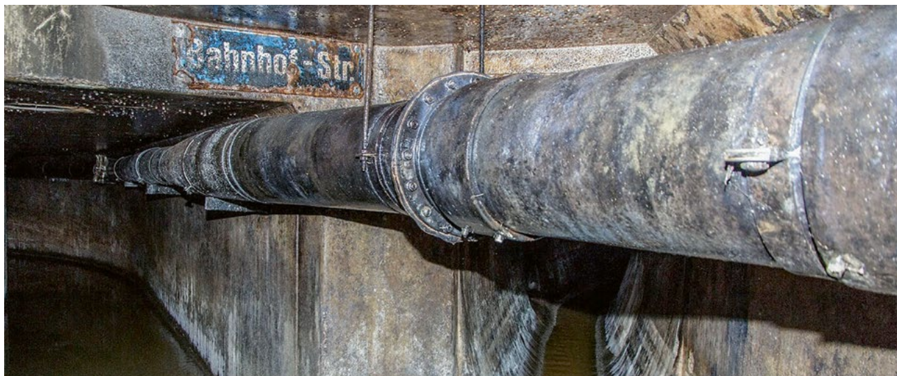
↑ Beneath the Bahnhofstrasse in Zurich, a sewer conveys wastewater to the treatment plant. Rainwater is channelled through a separate pipe.
