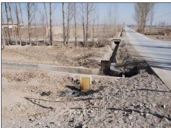
Figure 49: Small irrigation channels in the Sanqing district
