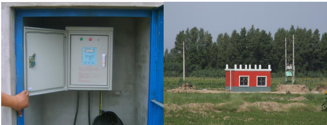
Figure 1 Monitored pumping well with IC-card [Kinzelbach 2013]. Using an IC-card, the user is allowed pump a specified quantity of water over a certain time.
