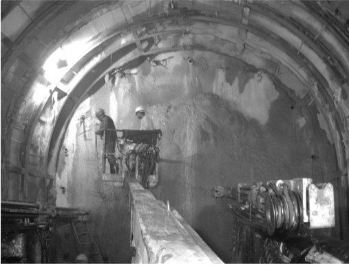
Figure 4. A typical situation during ongoing injection works. The steel pipes for injection are seen along the perimeter of the tunnel face.
