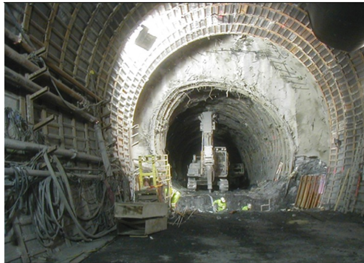
Figure 1. Squeezing rock reduces the tunnel cross section. This is shown in this photograph where re-profiling of a highly deformed cross section is taking place in the Saint Martin access adit (Lyon-Turin Base Tunnel).
