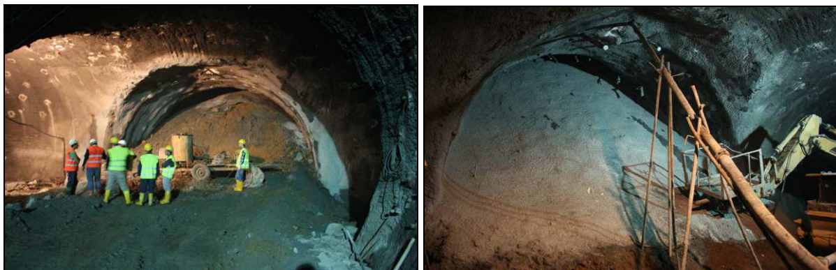
Fig. 6.2: Ayrilikcesme station – Little accident during Stair tunnel excavation
