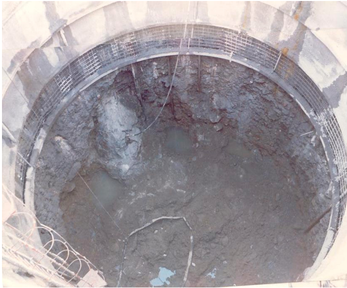
Fig. 1. Excavation of a large diameter drilled shaft (photo courtesy by Ulrich Hegg Eng. MSc., Milan).
