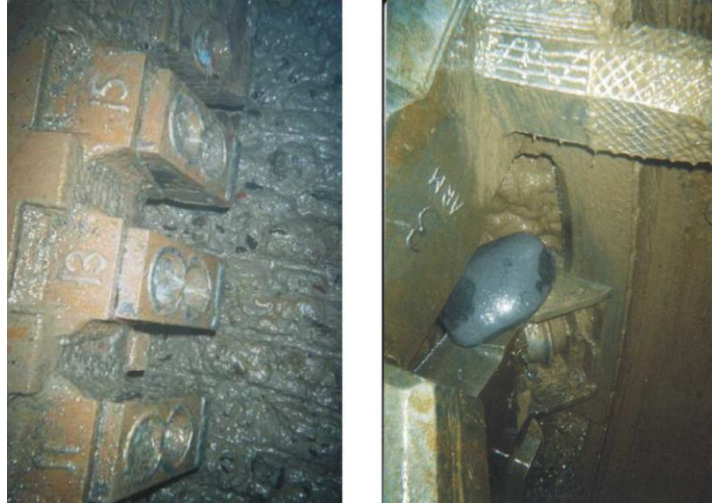
Figure 12. East Side CSO Portland, tunnel face (left) and boulder entering the excavation chamber (right)
