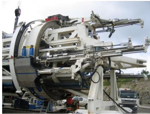
Figure 14: Permanent drill installation at the front end of the trailing gear behind the erector
