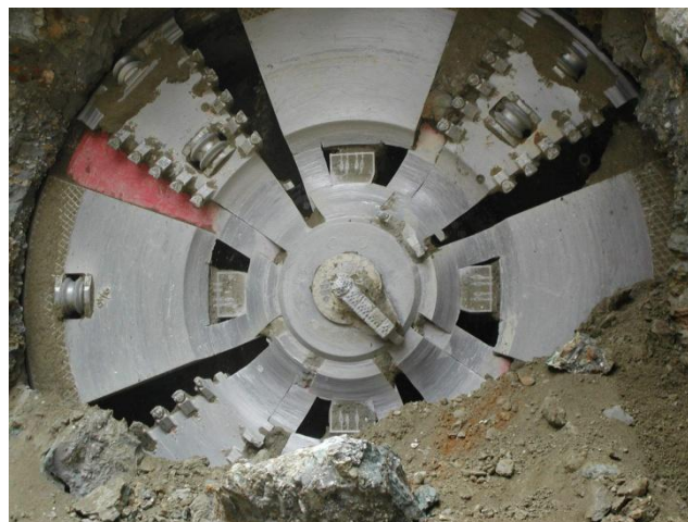
Figure 13. Cutterhead damage as consequence of broken cutter disc
