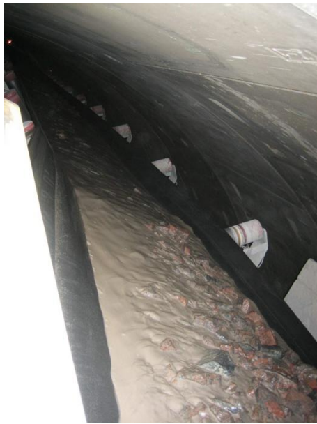
Figure 13: Water laden muck on gantry conveyor
