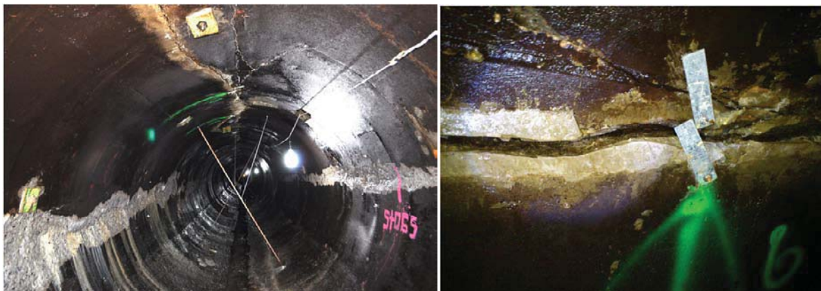
Figure 3. Stretch of damaged headrace tunnel and fracture detail
