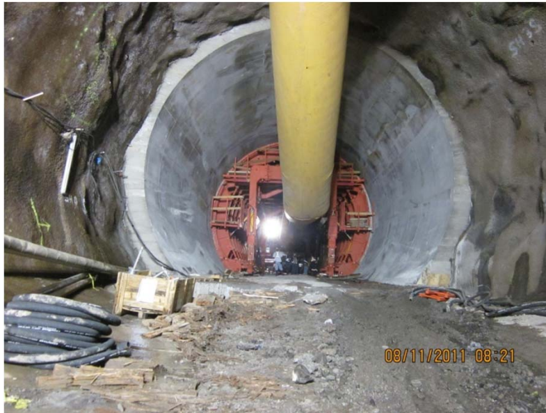
Realization of the final lining with cast in place concrete. Minimum thickness = 30 cm Reinforced with steel ribs (minimum dosage 35 kg/m 3 )
