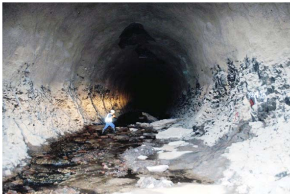
Lining (shotcrete) detachments probably occurred in the dewatering phase
