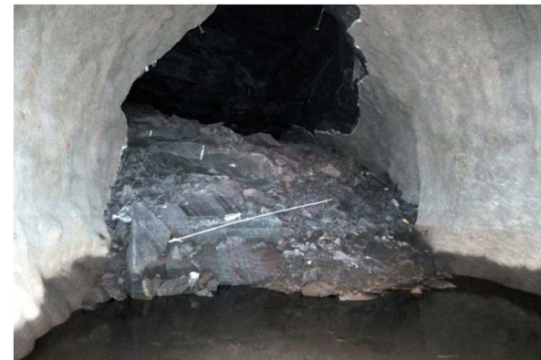
Complete obstruction of the tunnel section due to a collapse
