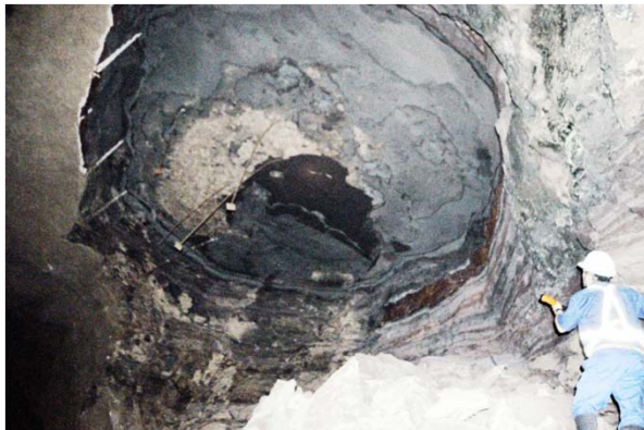
Collapses in tunnel roof controlled by rock-mass stratification. Sub-horizontal rock layers were separated by water-sensitive mudstone layers. Maximum collapses height: 5 m.
