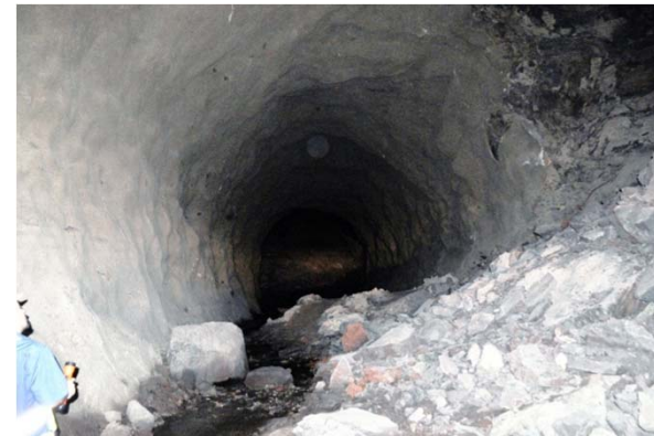
Collapses at tunnel walls probably occurred in the dewatering operation consequent to the main collapse.
