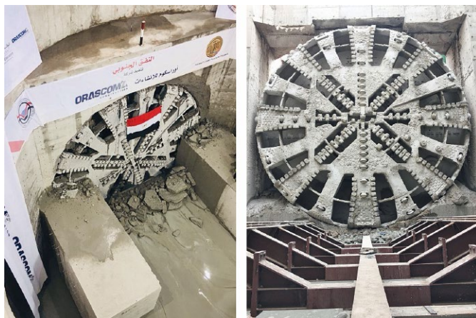
Fig. 14. South TBM breakthrough (left) and disassembly preparation at the second cell in the reception shaft for north TBM (right)
