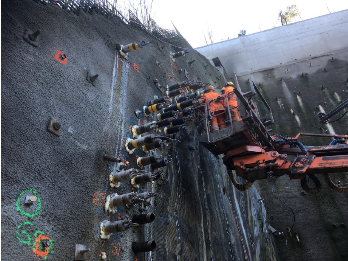
Figure 12. Steel tubes of the triple pipe umbrella (picture: courtesy of Implenia Switzerland).
