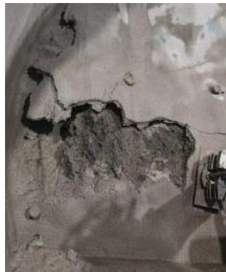
Figure 11. Splitting of shotcrete from the face
