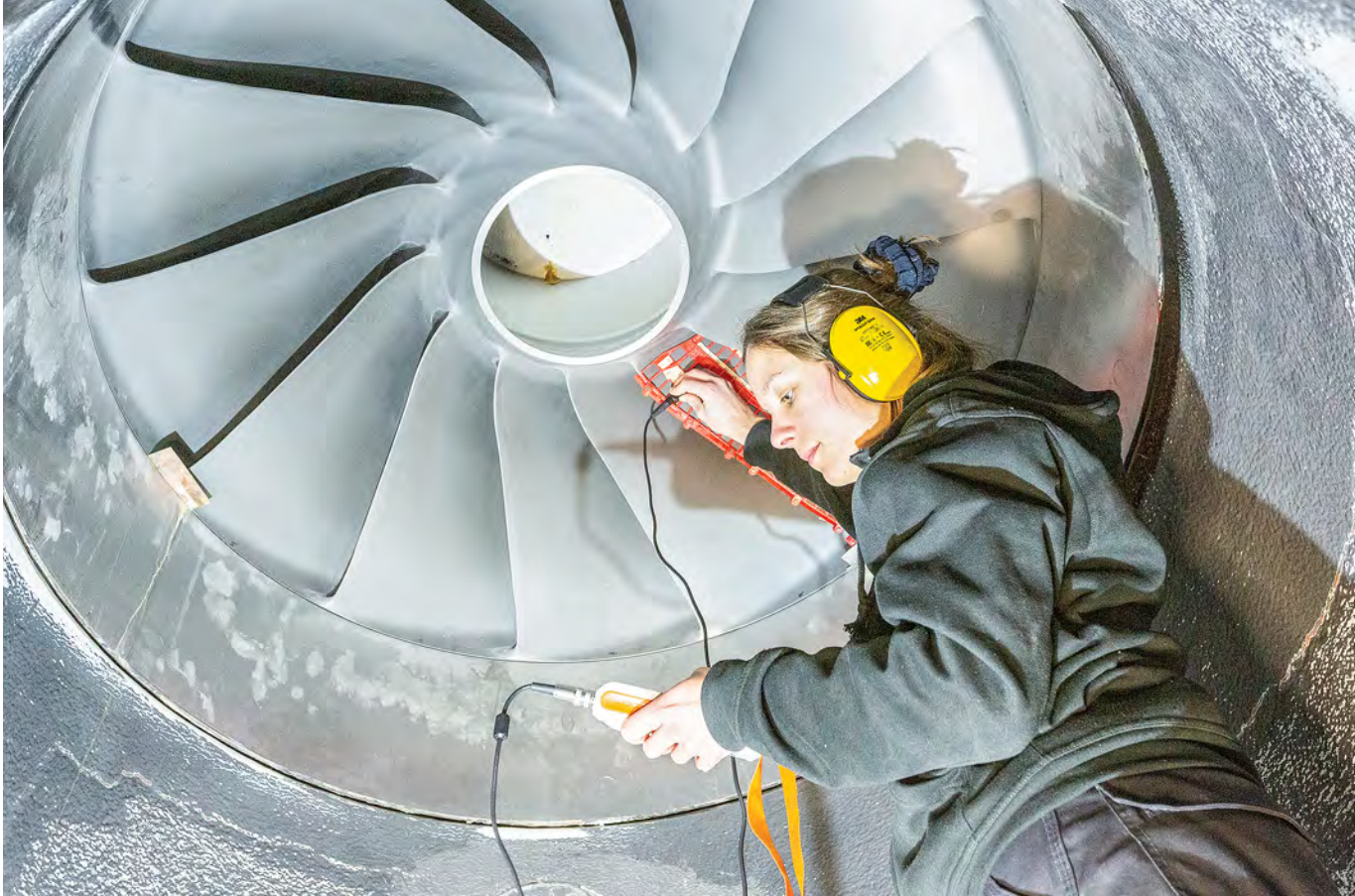
Fig. 5: Coating thickness measurement of the partly coated Francis turbine at Langenegg HPP.
