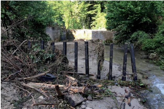
Accumulation of bed load and driftwood after the flood in June 2015 (Photo: Stadt Luzern)
