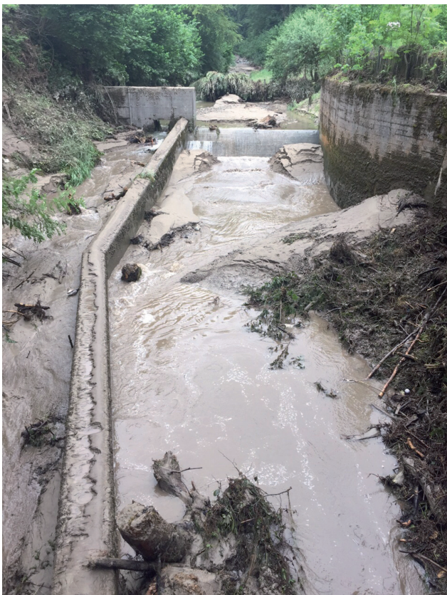
Accumulation in the intake area of the spillway tunnel (Photo: David Cathomas)
