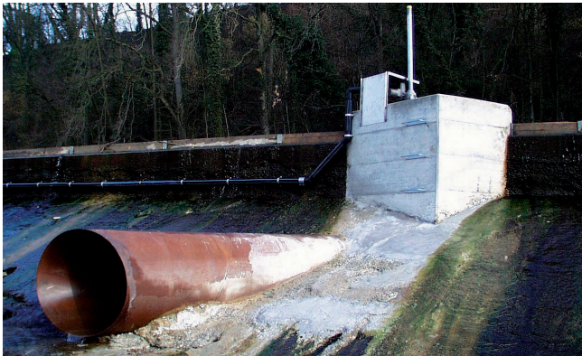
View of the outlet of the vortex tube at the hydropower plant Schiffmühle from the residual flow reach
