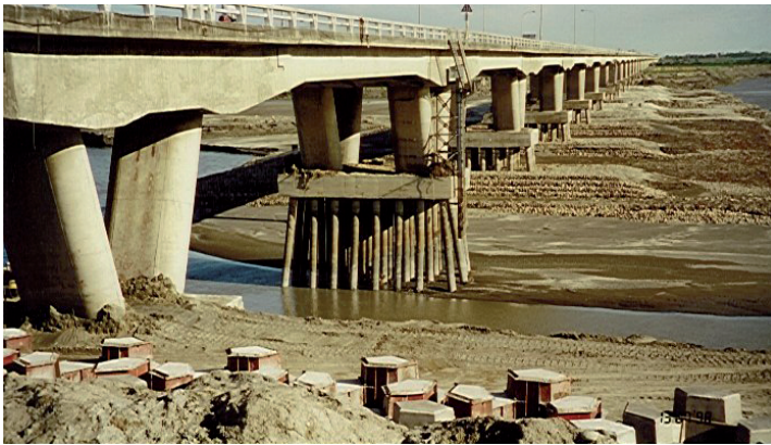
Fig. 1: Bridge pier scour in New Zealand (Melville and Coleman, 2000).
