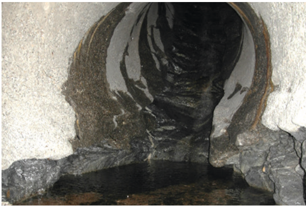
Up to a 2 m deep abrasion incision at the Val d'Ambrè SBT into the concrete lining and underlying rock (M. Müller-Hagmann)
