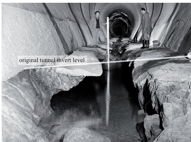
invert abrasion in Palagnedra sediment bypass tunnel, Ticino, Switzerland
