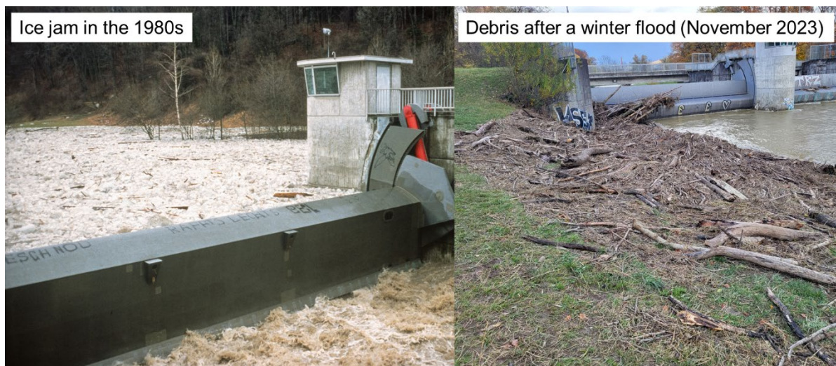
Fig. 1: Ice weir on the Sihl river with ice jam and floating woody debris
