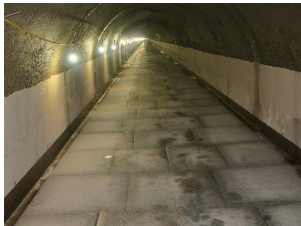
Fig. 1: Granite invert lining of Mud Mountain SBT (Source: US Army Corps of Engineers)
