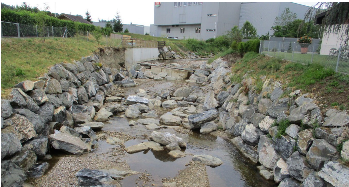
Fig. 1: Remnants of a block ramp in Zell (LU) after its failure (May 2023).
