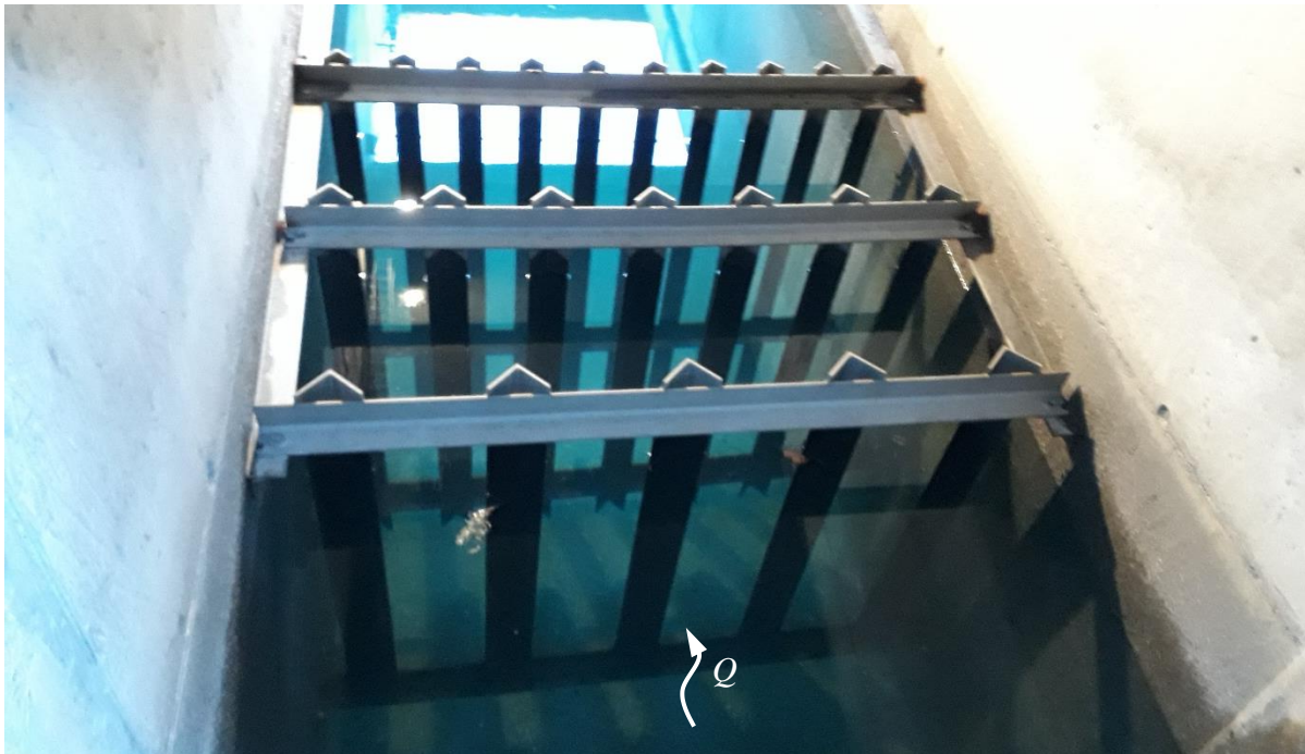
Fig. 1: Three rows of TRs with vertical, v-shaped bars at HPP Susasca (Source: VAW)
