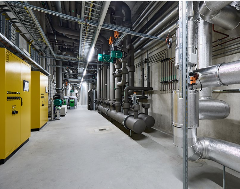
Heating and cooling supply centre on the B floor
