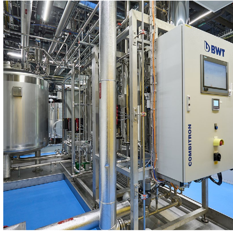
Grey area outside the GMP clean room on the B floor
