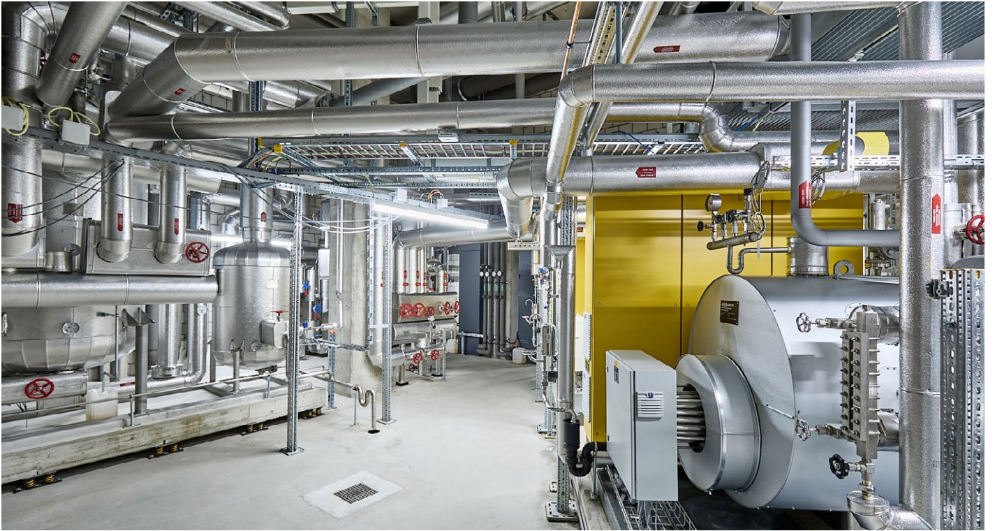
Steam centre on the B floor
