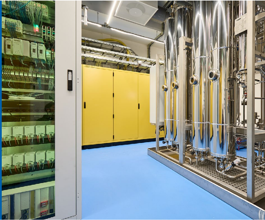
Grey area outside the GMP clean room on the B floor
