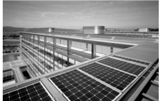
Solar panels on the ETH building HCI
