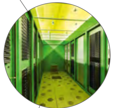
High Performance Computer facility at ETH.
