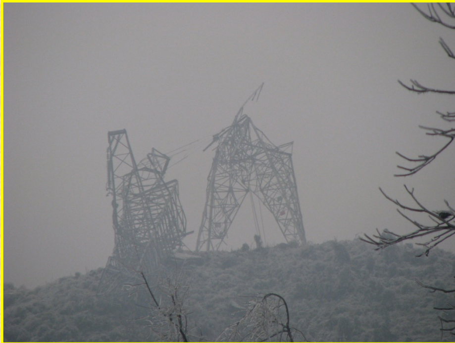
Failure due to cable disconnect
