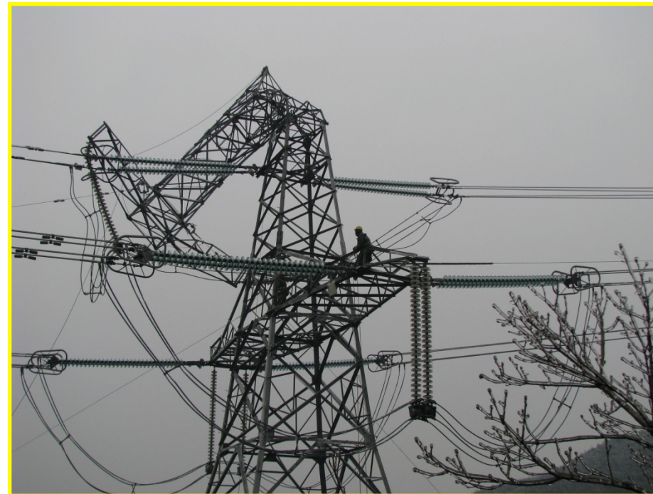
Failure due to unbalanced tension in cables
