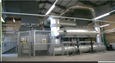
Combined heat & power engine (CHP)
