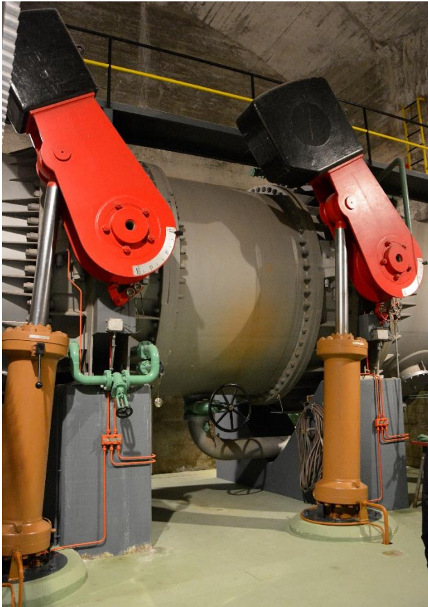
Butterfly valves (penstock)
