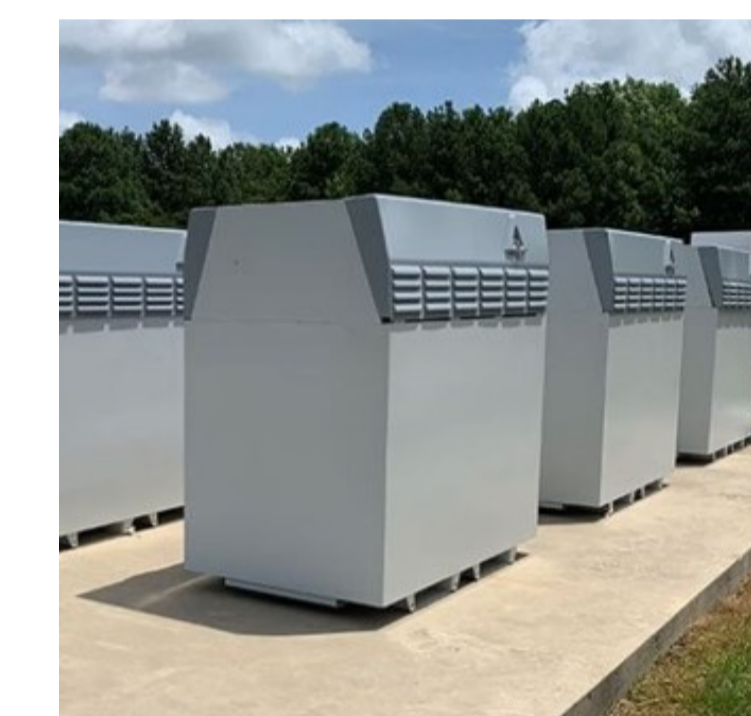
0.5 MWh, Alabama, USA Operator: Southern Company / EPRI
