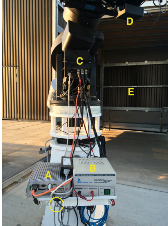
Figure 4: Overview of electronics: main power switch (circle), remote computer (A), power adapter GM4000 mount (B), router (B), GM4000 control box (C), Delta-T control box (D), (handles to push/pull dome (E)).
