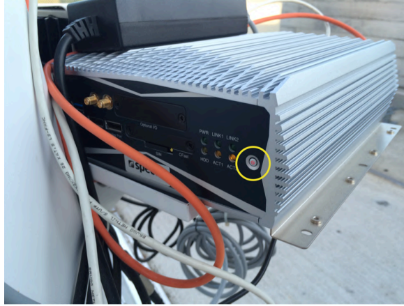
Figure 9: Power switch of the remote computer (circle).
