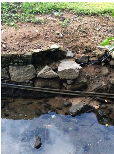
Figure 24: A permeable bank bed in a poor condition (Rivière Maintry, own source, 14/04/2019).
