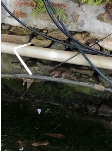
Figure 71: Rat walking on pipes (Rivière Maintry, own source, 14/05/2019).
